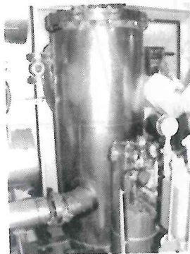
Mixing Column/ Buffer Tank
