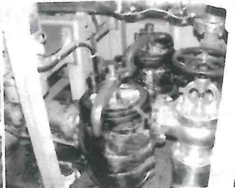
Supply Pump Suction Filters
